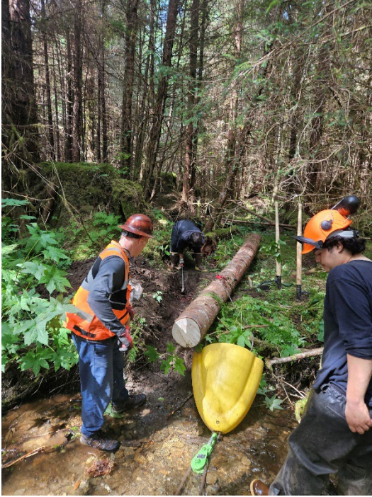
A trench in the bank is prepared to receive a log in July. The log will extend into the channel to promote scour, gravel sorting, and pool formation improving habitat complexity for trout and char.
