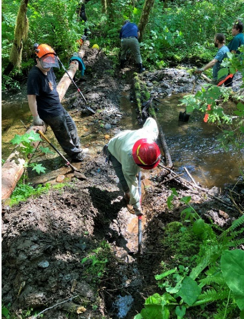
Partners dig a trench in the stream bed and bank prior to placing a log across the channel to form a pool in June.
